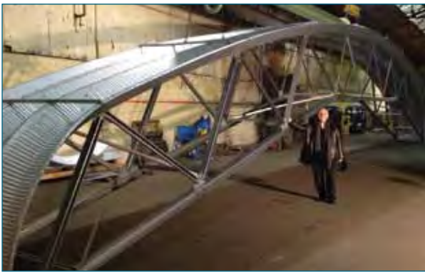
Once the infrastructure is completed, bolt the panels together to complete one section, which is really three sections joined together.
