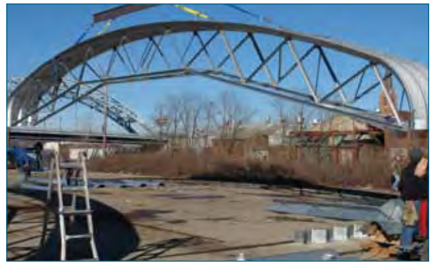
When the sections are completed, lift the roof up with a crane or a boom.
