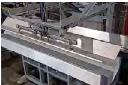
The finished roof panel is automatically loaded onto a conveyor which moves the panel into the crimping machine.
